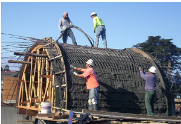
After the shotcrete was sprayed onto the sheet metal covering, crews burned in a "buttery" finish with small fresnos.
