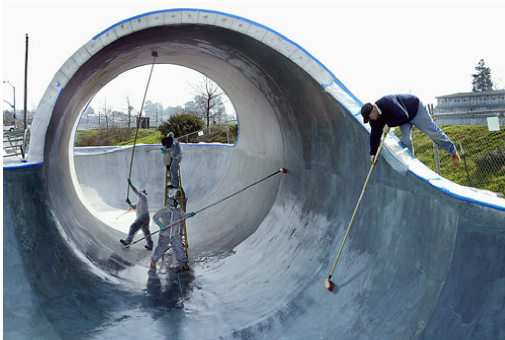
A crashing concrete wave created with acid stain and sandblasting is a piece of public art paying homage to Santa Cruz's surfing culture.
